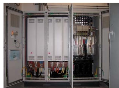
Interior View 1.6MVA Unit @ 480V
